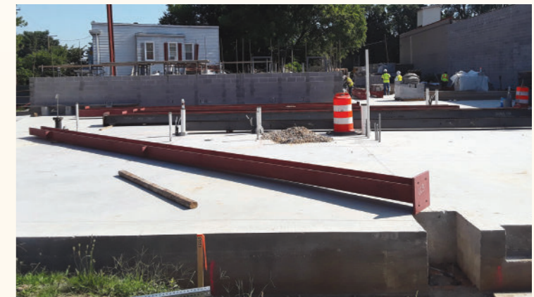
In July, steel beams were put up on our new Southeast Center! At our new center on Good Hope Road SE, we will welcome and care for thousands more men, women, and children.
